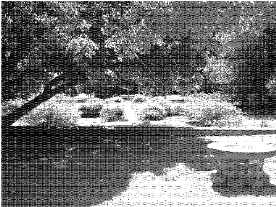
Sharp's construction of a three-foot wall that divided the lawn from the garden. (Cathy Kinney, October 2010).
