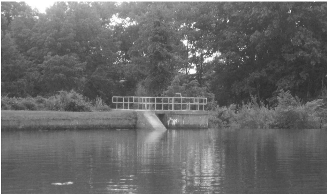
Image 3: Stop-log section of the spillway. Field photograph taken by HAER recording team, summer 2009.
