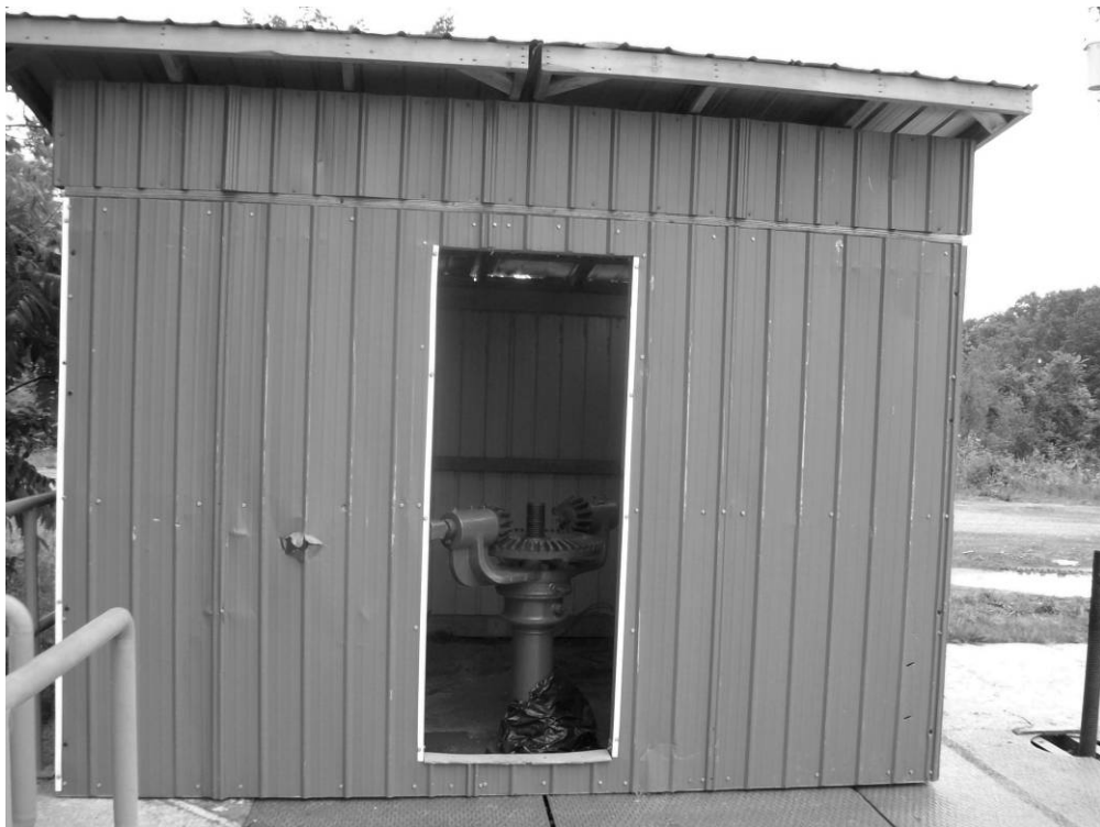
Image 3: Shelter over sluice gate valve. Field photograph taken by HAER recording team, summer 2009.
