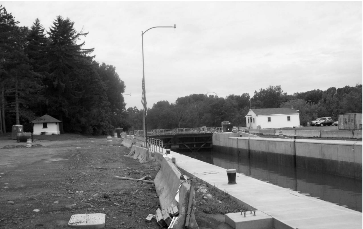
Image 1: Overview of lock with storehouse to left of chamber and lockhouse to right. Field photograph taken by HAER recording team, summer 2009.
