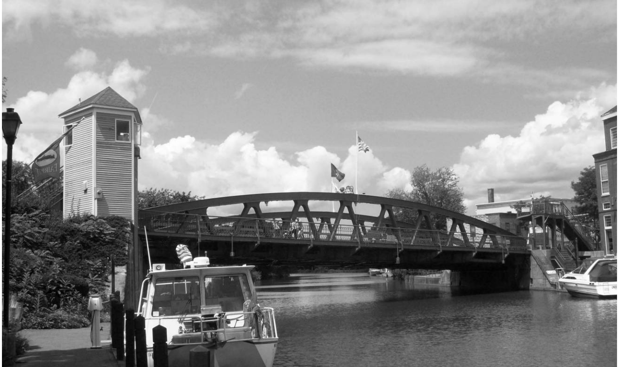
Image 1: Elevation of Fairport Lift Bridge with control tower at left. Field photograph taken by HAER recording team, summer 2009.
