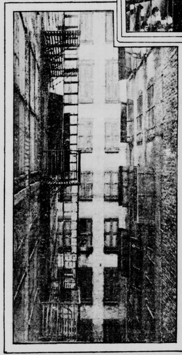
THE FIRE-ESCAPE ON THE TRIANGLE-WAIST BUILDING BEFORE THE FIRE, DURING WHICH IT COLLAPSED CAUSING MANY DEATHS
