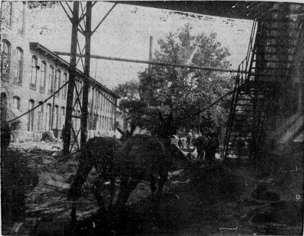
Above photo shows the grading work going on between the Roanoke Mills Company plant No. 1 buildings as hundreds of employees worked day and night to get the mill running again. Parts of the mill started up this week. More is expected to start soon, with the entire mill getting underway in a very short time.
